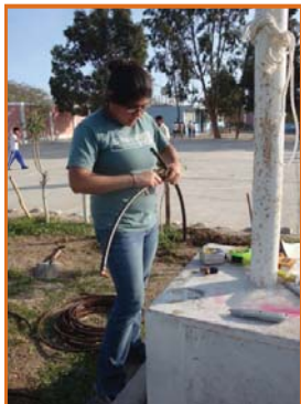
Cynthia Castro, civil engineering senior, helps prepare the irrigation system that was built at the only school in Santa Cruz, Peru.
