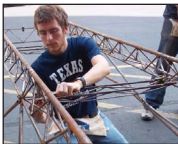
ASCE Steel Bridge Co-Chair Jeffrey Stump helps assemble the steel bridge constructed entirely by students.
